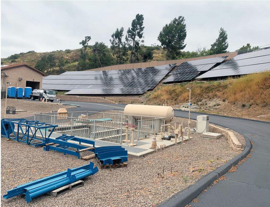
The 278 kW Lower Moosa Canyon photo-voltaic solar array.
