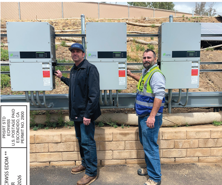
Roy Rutherford, VCMWD pumps, motors, facility and fleets supervisor and Ash Padilla of SunRenu, energize the 278 kW Solar Array at the Lower Moosa Canyon Water Reclamation Facility (Moosa) owned and operated by the Valley Center MWD, located near Circle R Drive and Old Highway 395.
