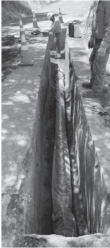
VCMWD workers replacing a water pipe. Some of the pipes in the system are 50 or 60 years old.
